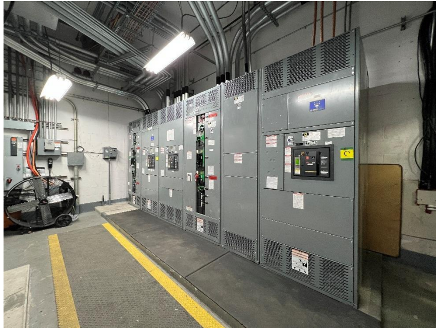
Hospital Electric Panels
